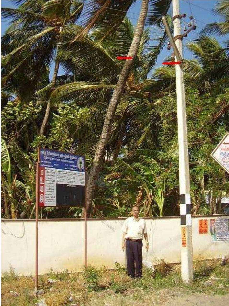
Photo 1. Shows the tsunami mark on the coconut tree and metallic part on the electric lamppost, which have been corroded. The points have been marked in red. This gives a clear idea of Tsunami height.
