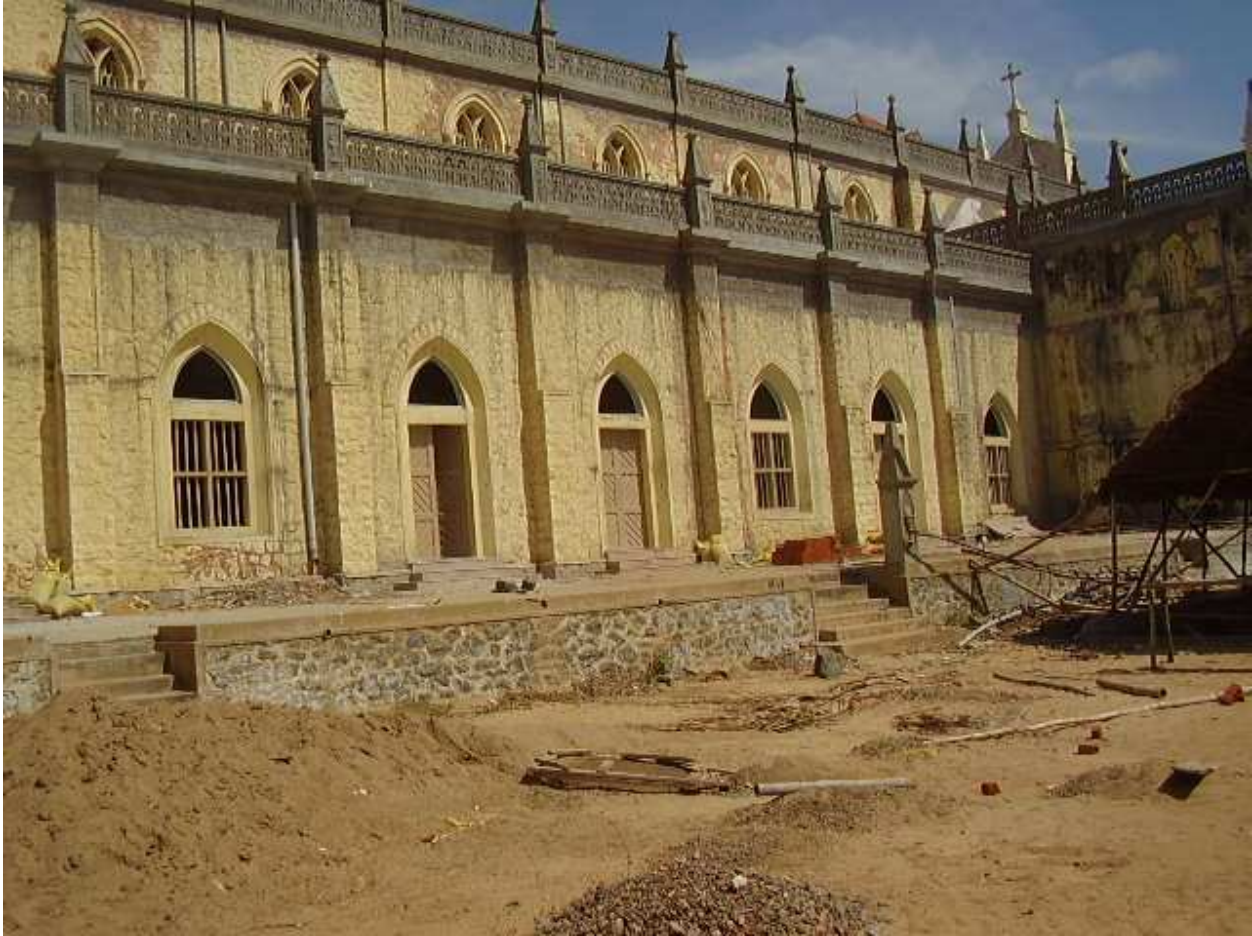
Photo 4. The repairs on first floor indicate damage during tsunami and the level of Tsunami height.
